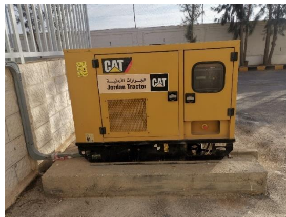
Figure 2: Diesel Generator Onsite
