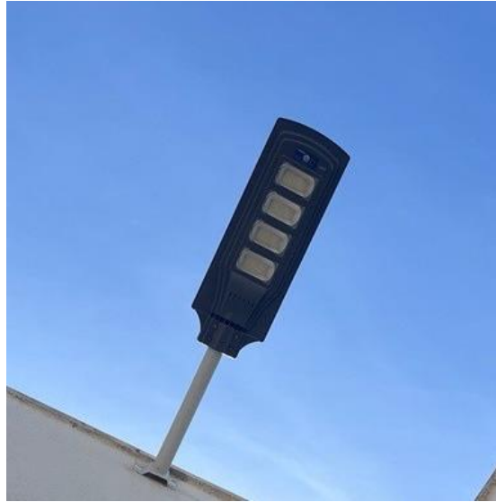
Figure 8: Solar lighting onsite
