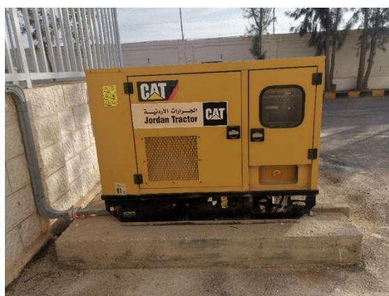
Figure 2: Diesel Generator Onsite
